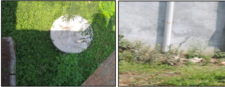
Fig. 8 Sewage Tanks in the college
